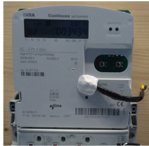
Fig. 5. Optical sensors as attached to a static meter
