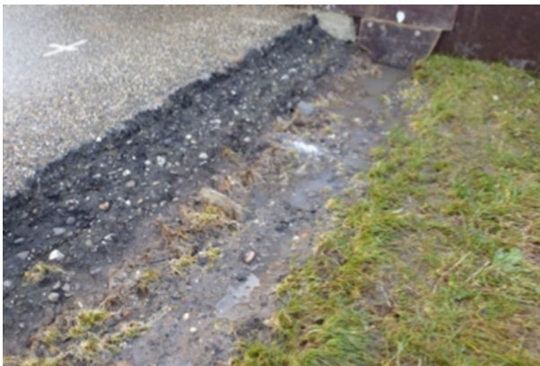
Fig. 3 Damaged transition present before the experiment in Millingen aan de Rijn started (Bakker et al. 2013). The damaged grass sod highly influenced erosion development on the landside transition
