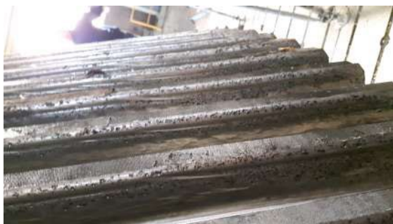
Fig. 4. Largest gear with damage.
