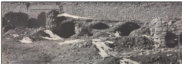
Figure 3. The collapsed brick made roof of The Deir`e Kaj caravanserai. Resource: Kiani and Kleis, 1373.
