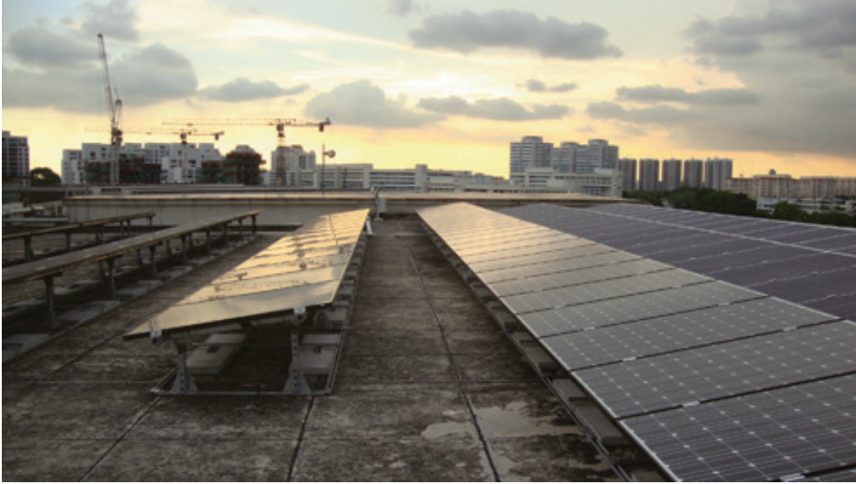
Fig. 7.1. SERIS' demonstration PV system, located at the National University of Singapore (NUS) campus.
