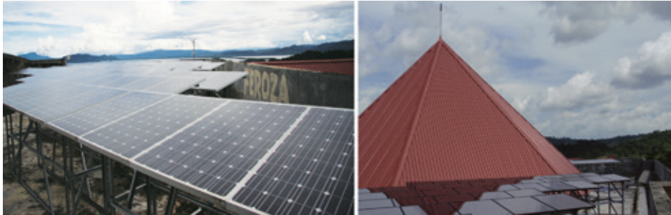
Fig. 5.4. Photo of the rack-mounted mono-crystalline silicon PV modules (left) and amorphous silicon PV modules (right) on the roof of the district office in Jayapura.
