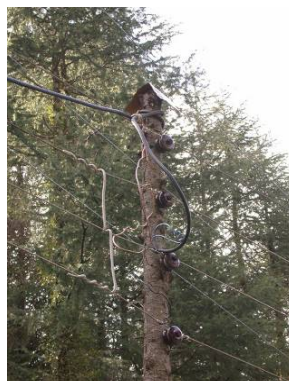
Photo 5.2 Bhuiira Jams, electricity supply
