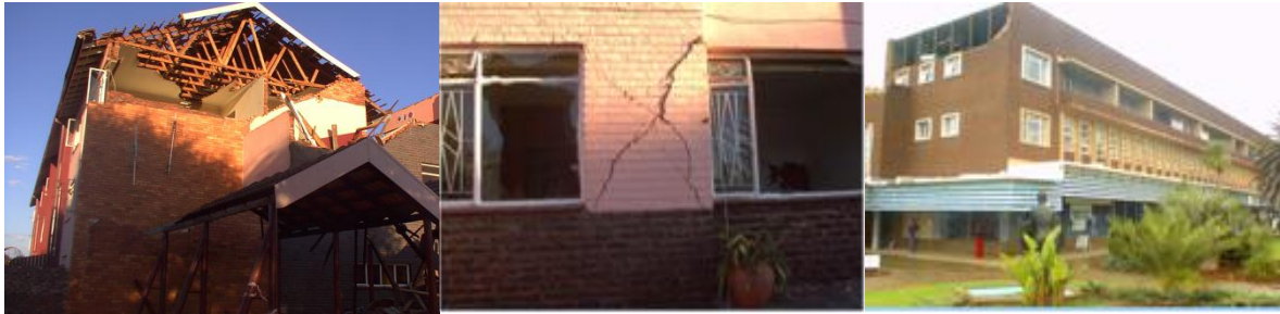
Figure 1: Building failures due to earthquakes in Stilfontein, South Africa (March 2005)
