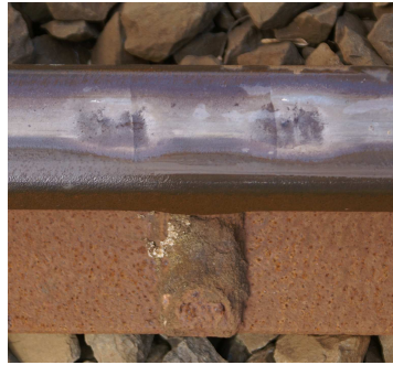
Figure 1: Squats initiated at a thermite weld
