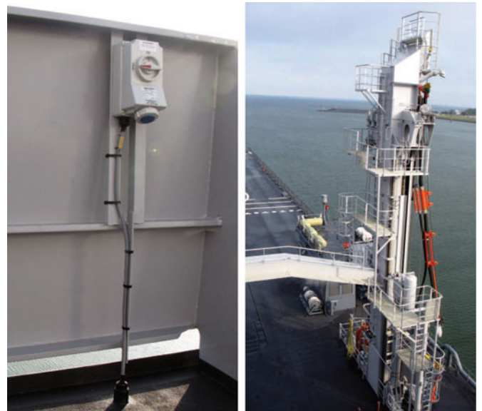
Fig. 3. Power outlet and installation for RAS.
