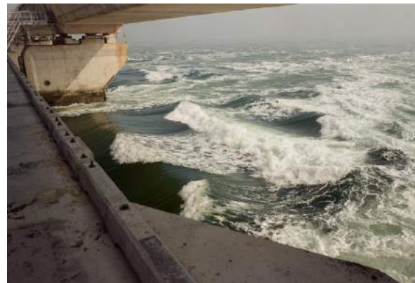
Figure 2 A Barrier opening of the Eastern Scheldt storm surge barrier (source: Beeldbank RWS).
