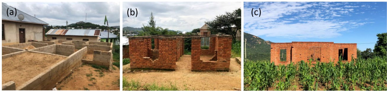
Fig. 3 Incomplete sand block (a) and burnt brick (b and c) masonry buildings. Photograph by Giulia Jole Sechi, Iringa, Tanzania 2021
