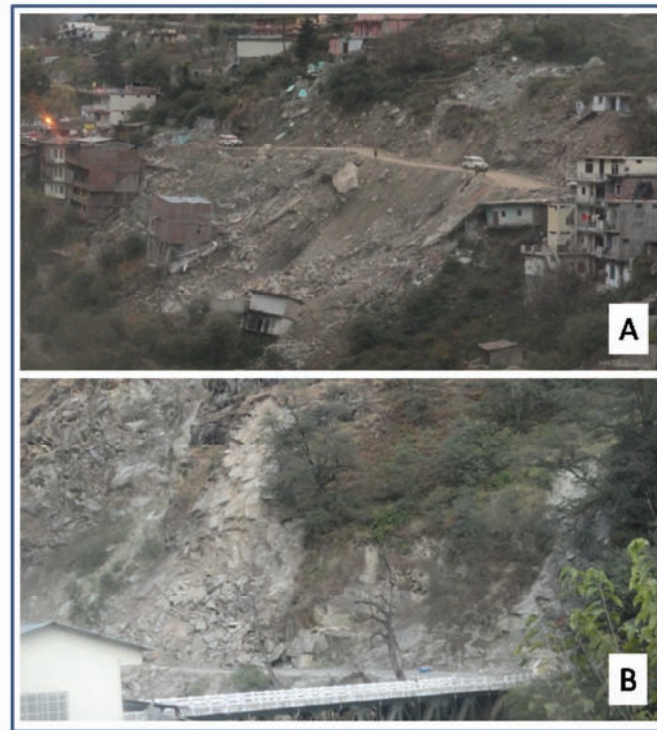
Figure 4.6 Landslides occurring along the road corridor, (A) a large rock-cum-debris slide damaging the houses and the road (B) a rock slide blocking the road partially
