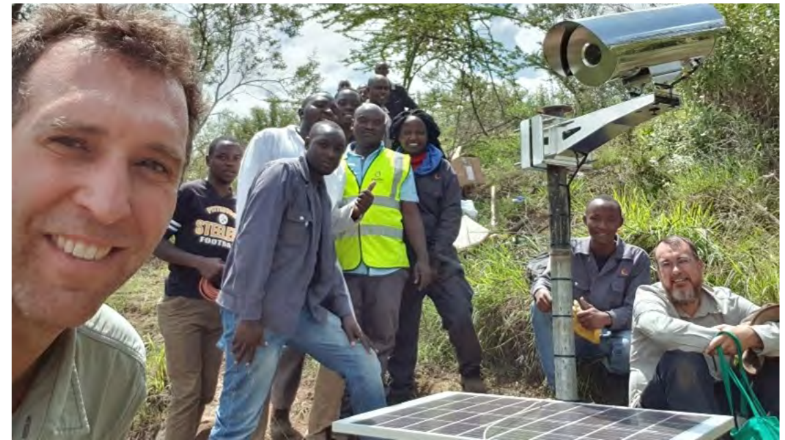
Figure 6: Installation of ground-based thermal cameras for the long-term monitoring of geothermal fumaroles.
