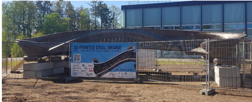
Fig. 1. The MX3D Bridge during the commissioning period at the University of Twente.
