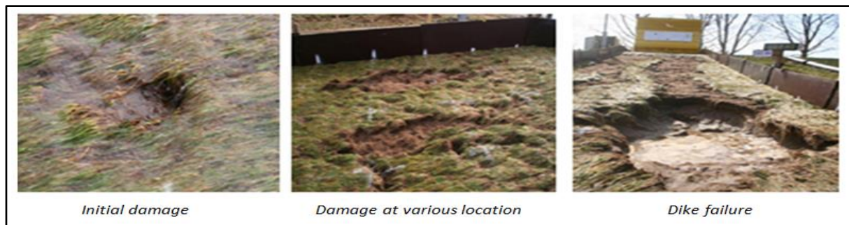
Figure 1.5. Initial damage, damage at various locations and dike failure (Van Hoven et al., 2013)
