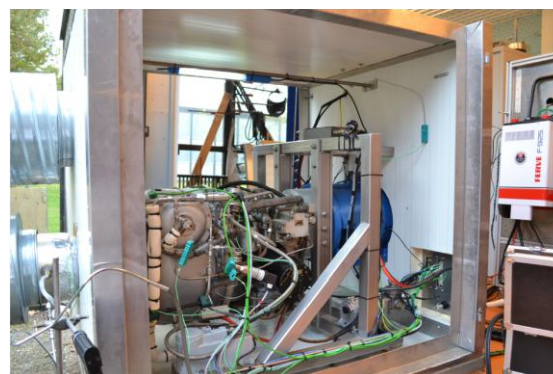
Figure 2. DG4M-1 micro gas turbine in noise absorption box.
