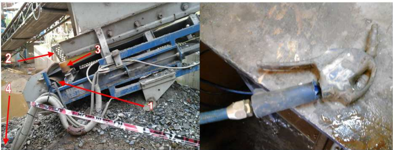
Fig. 4. Left picture. Section of the conveyor belt involved in the injury as observed by the investigators: 1. Tail pulley of the conveyor belt; 2. Side fixed guard mounted only on the left side of the conveyor belt; 3. Load carrying roller replaced during the operation; 4. Position of the air gun after the accident. Right picture: air gun involved in the accident
