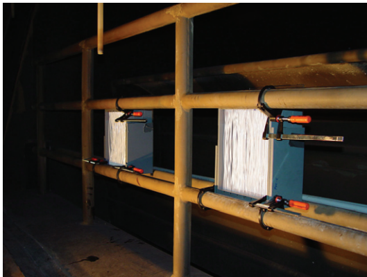
Figure 1: Membrane test modules in an actual flue gas duct of a waste to energy plant for capturing water from flue gas
