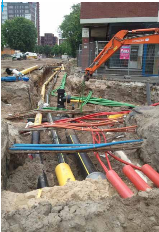
FIG.1 Subsurface utility challenge: unraveling the subsurface cables and piping spaghetti
